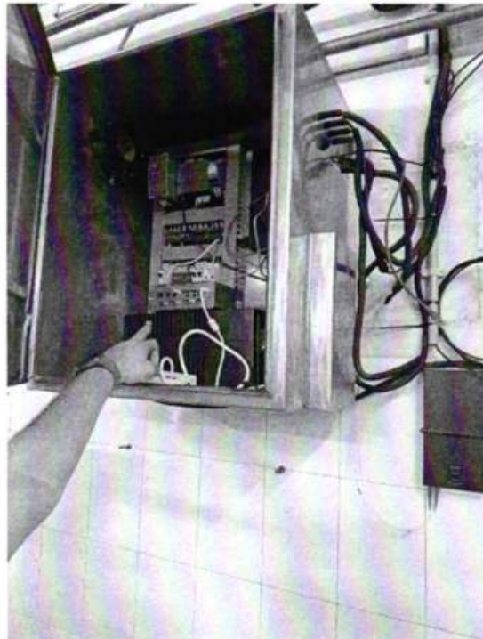
Image 2 Interior of the controller enclosure showing the PLC with I/O modules, DIN-rail power supply, terminal blocks, circuit protection, industrial edge computer, UPS and cooling fan
