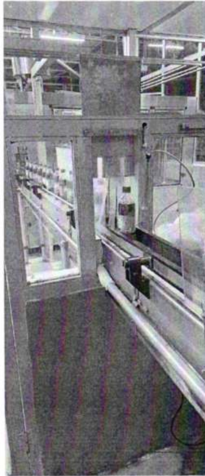
Image 1 — The Vendor's barcode scanning enclosure installed over the production line conveyor
