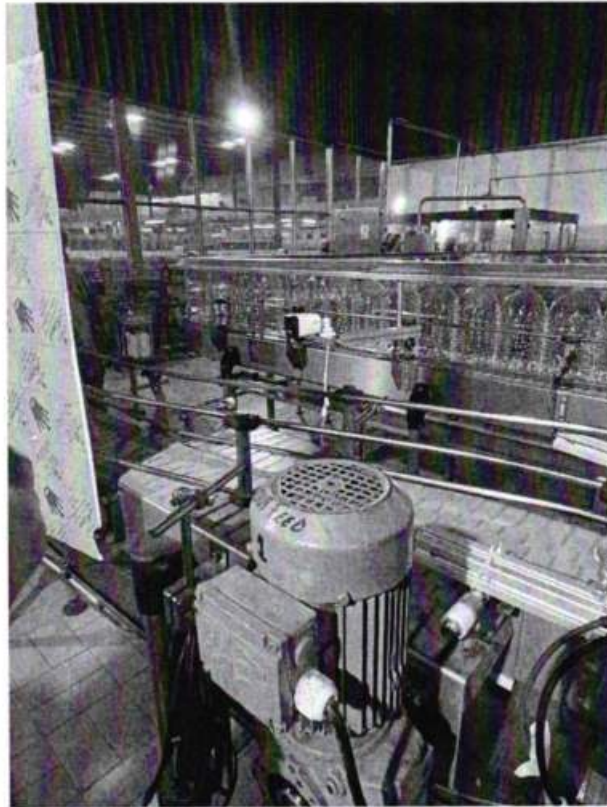
Image 4 AI vision camera (IP bullet camera) mounted over the outfeed conveyor
