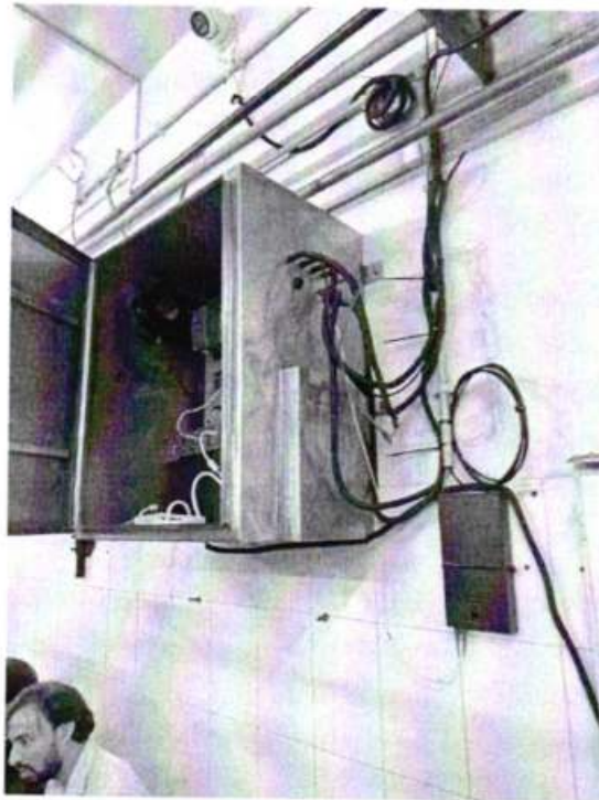
Image 1 Stainless-steel waterproof controller enclosure with the camera mounted above to monitor the barcode reading position, conduit cabling and fibre-optic termination
